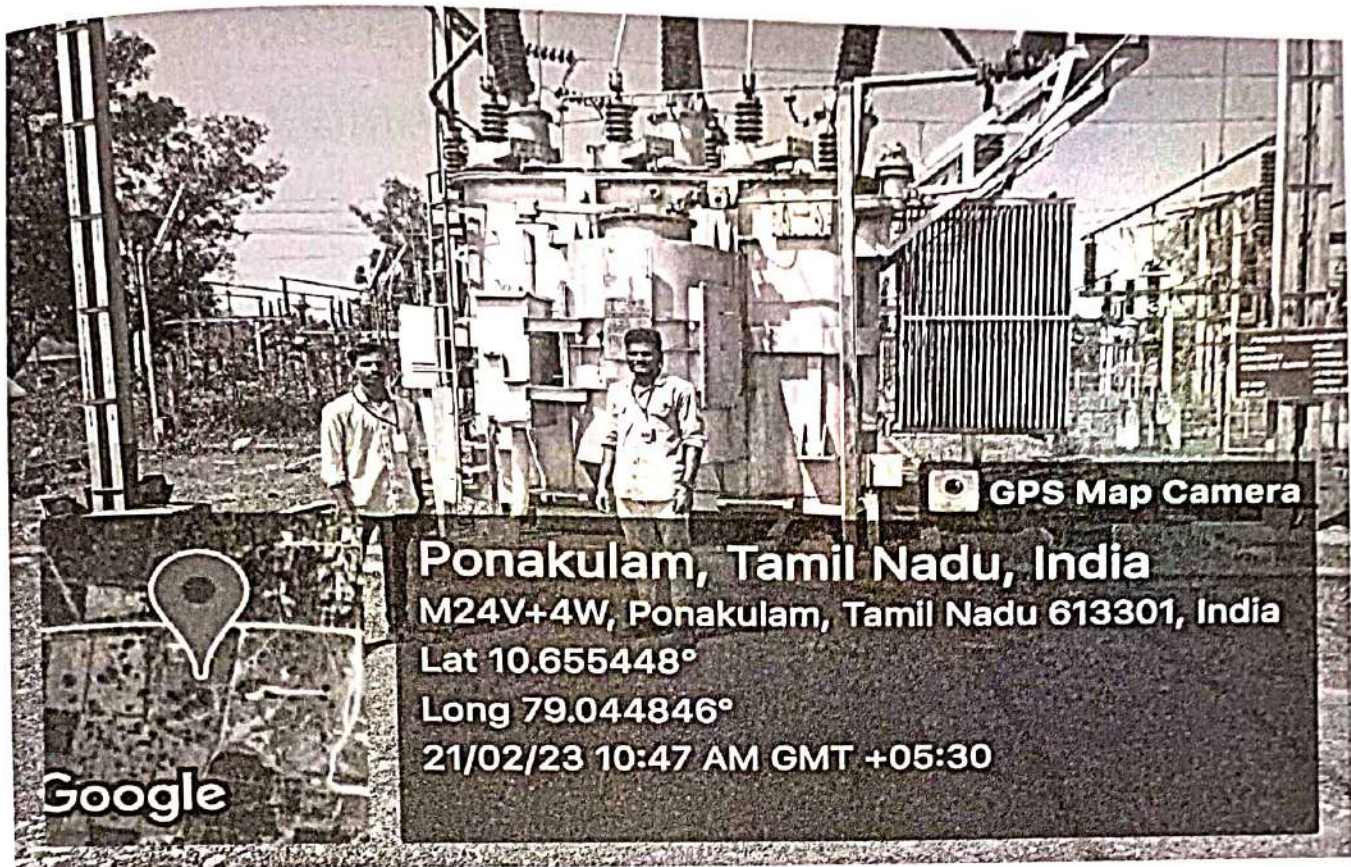
Figure 3:Field visit at 110/11KV POWER TRANSFORMER
